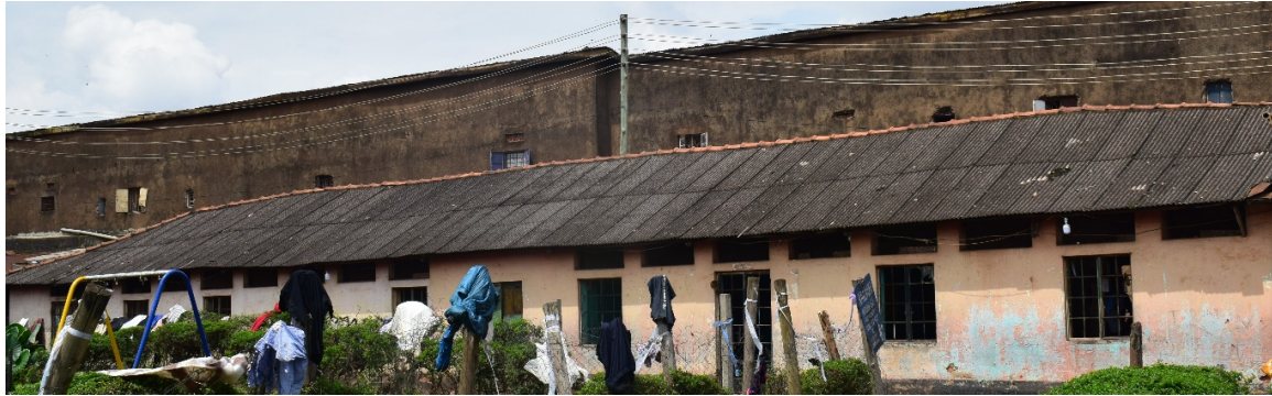
Fig. 32: Existing classroom block with asbestos roof covering:- Waiting for more Funds to implement renovation works at the school block, (replacement of the asbestos with an environmentally and health safe material, installation of new windows and doors, plastering and painting of the wall structures, estimated budget UShs. 160,000,000.
